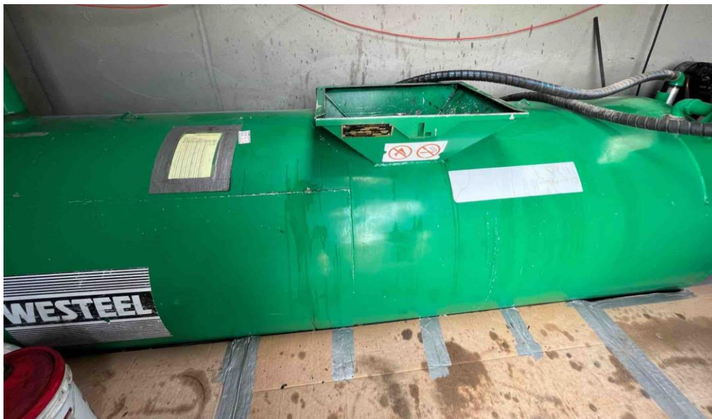
Storage Tank and Secondary Containment
